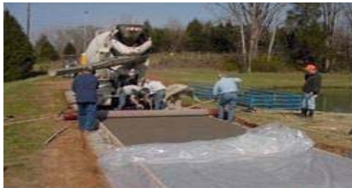
Figure 10. Pervious concrete being poured, consolidated and covered with plastic sheeting. Photo courtesy of the National Ready Mix Concrete Association.
