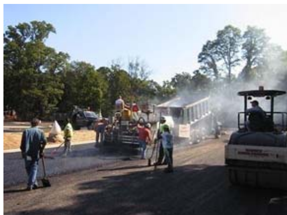
Figure 15. Porous asphalt installation for a Villanova parking lot. Photo courtesy of the Villanova Urban Stormwater Partnership.
