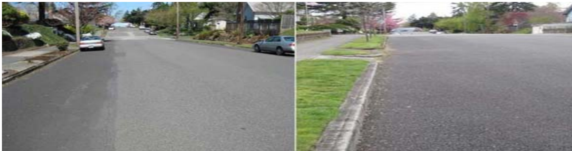
Figure 13. A curb to curb installation of porous asphalt (left) and an installation of porous asphalt in the parking lanes and conventional asphalt in the drive lanes (right). Photo courtesy of the Portland Bureau of Environmental Services.
