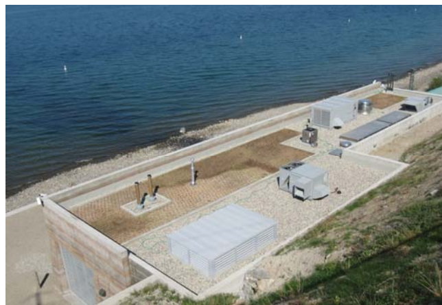
Figure 3. Cedar Creek pump station green roof, Kelowna
